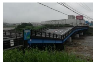
Damage to the Kise River Bridge (Numazu City, Shizuoka Pref.)
