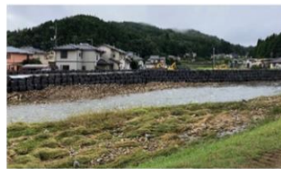
Levee Broken (Tajihigawa River)
