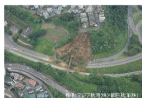
Slope collapse at Zushi Interchange (Zushi City, Kanagawa Pref.)
